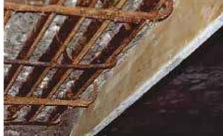
1. Spalled beam and rusted rebar
