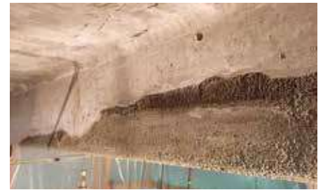
4. Patched concrete on coated beam
